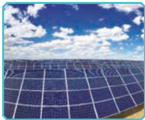
Xinjiang Hami Yaohui Large-scaled Solar Power Plant
