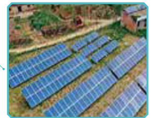
Anhui Funan Solar Energy Poverty Alleviation Project
